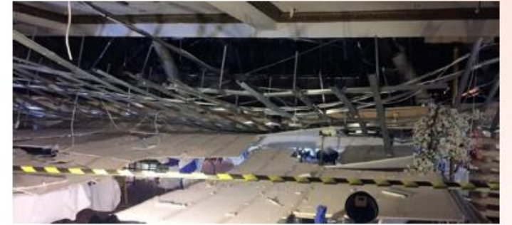
Figure 3. Inadequate fixings. Picture credit: West Midlands Ambulance Service
