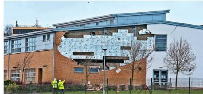
Figure 1. Incorrectly fixed cavity wall ties and omission of lateral restraint fixings.
